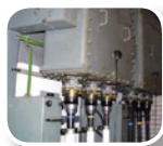
Power sensitive equipment
